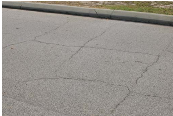
Figure 2.4: Pattern cracking of concrete pavement (LGAM, 2011)
