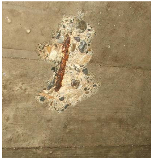
Figure 2.1: Effects of spalling, exposure of steel rebar (Buell, 2009)
