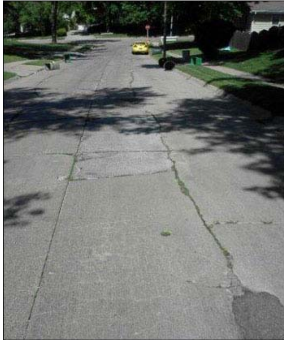
Figure 2.2: D-Line cracking at joints of slab (Omaha, 2012)
